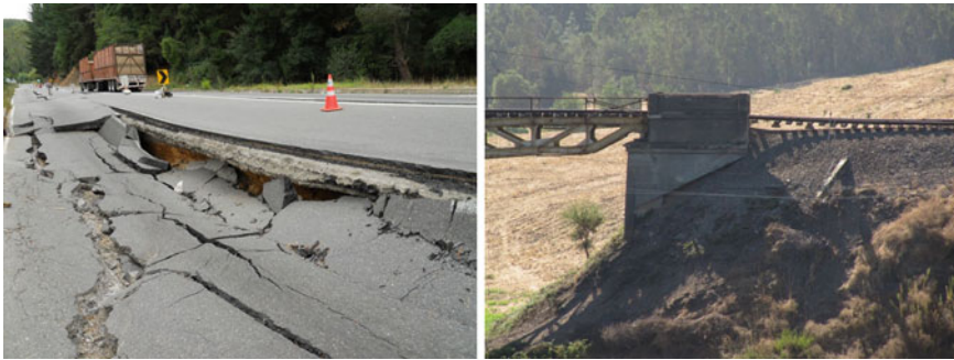
Fig. 1.35 Ground failure in a highway ( left panel ) and extensive settlement in a railroad bridge abutment ( right panel ) during the 2010 Maule, Chile earthquake (EERI Earthquake Photo Gallery)
