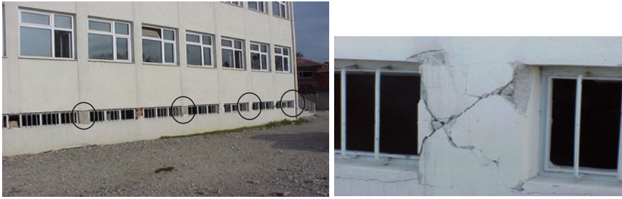
Fig. 7.19 Short column failures in a school building after the 1999 Düzce earthquake. Picture on the right shows detailed shear damage from one of the short columns
