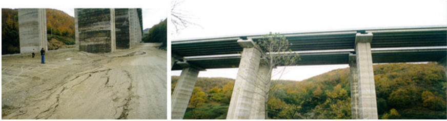
Fig. 1.34 Fault trace running across the Bolu Viaduct piers ( left ) and the damage caused at the deck structure due to static differential movement of the piers along the ruptured fault
