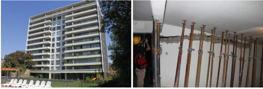
Fig. 7.30 Shear wall damage at the ground story of a modern concrete building during the 2010 Chile earthquake (M 8.8)
