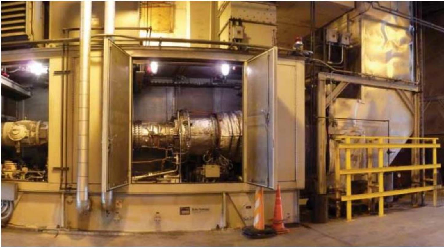
CHP system—gas turbine (center), with hot gases heading to heat recovery steam generator (right).
